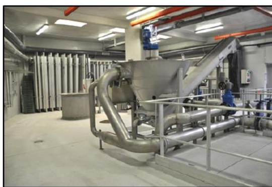
Station de pompage
