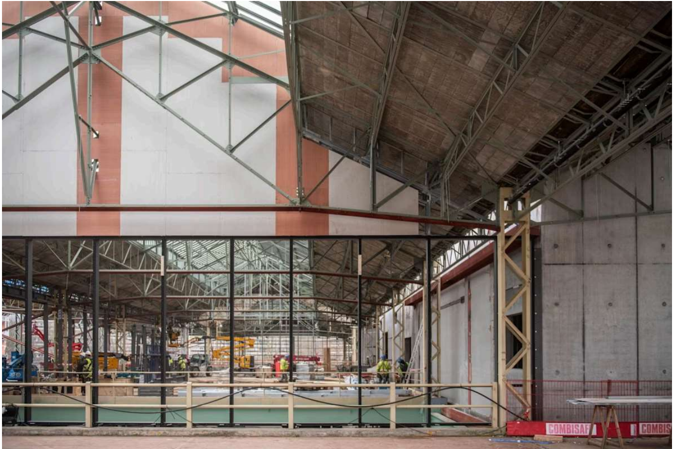
Work under way at the KANAL-Centre Pompidou, designed by Sergison Bates, noAarchitecten and EM2N © Bart Grietens
