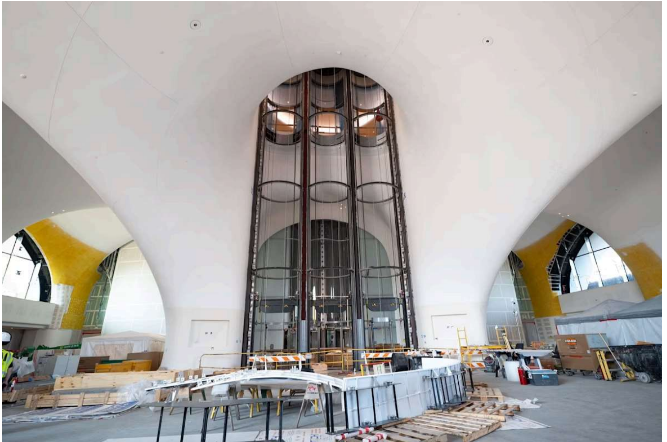
The lobby at the Lucas Museum, designed by MAD Architects, during construction
